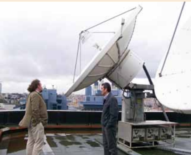
Intorel's Visionic can directly or remotely manage an entire network of satellite and broadcasting devices — regardless of the size and complexity.
